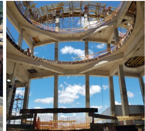
SPRAY 3 Villa Rodríguez Industrial Complex San José · Uruguay
