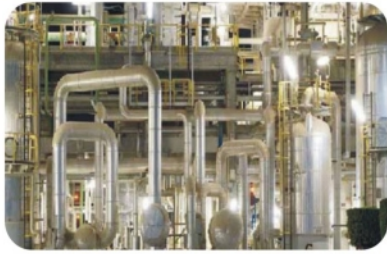
Water Piping System
