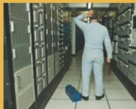
Server and communications facility
