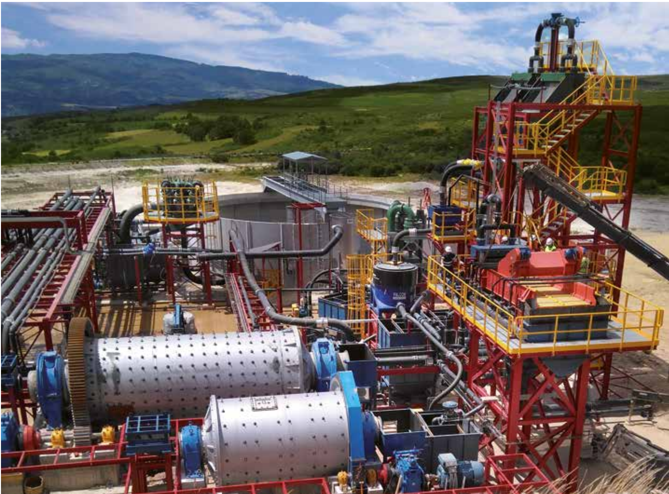
Mine ore beneficiation plant
