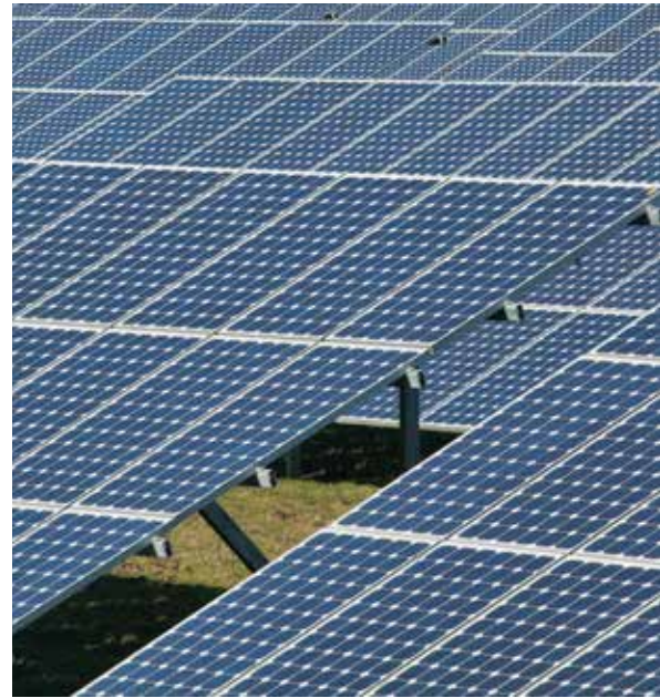
Intipampa Photovoltaic, Peru
