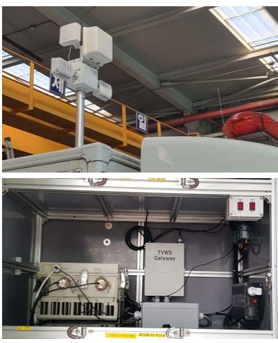
Firetruck Mobile Base Station
